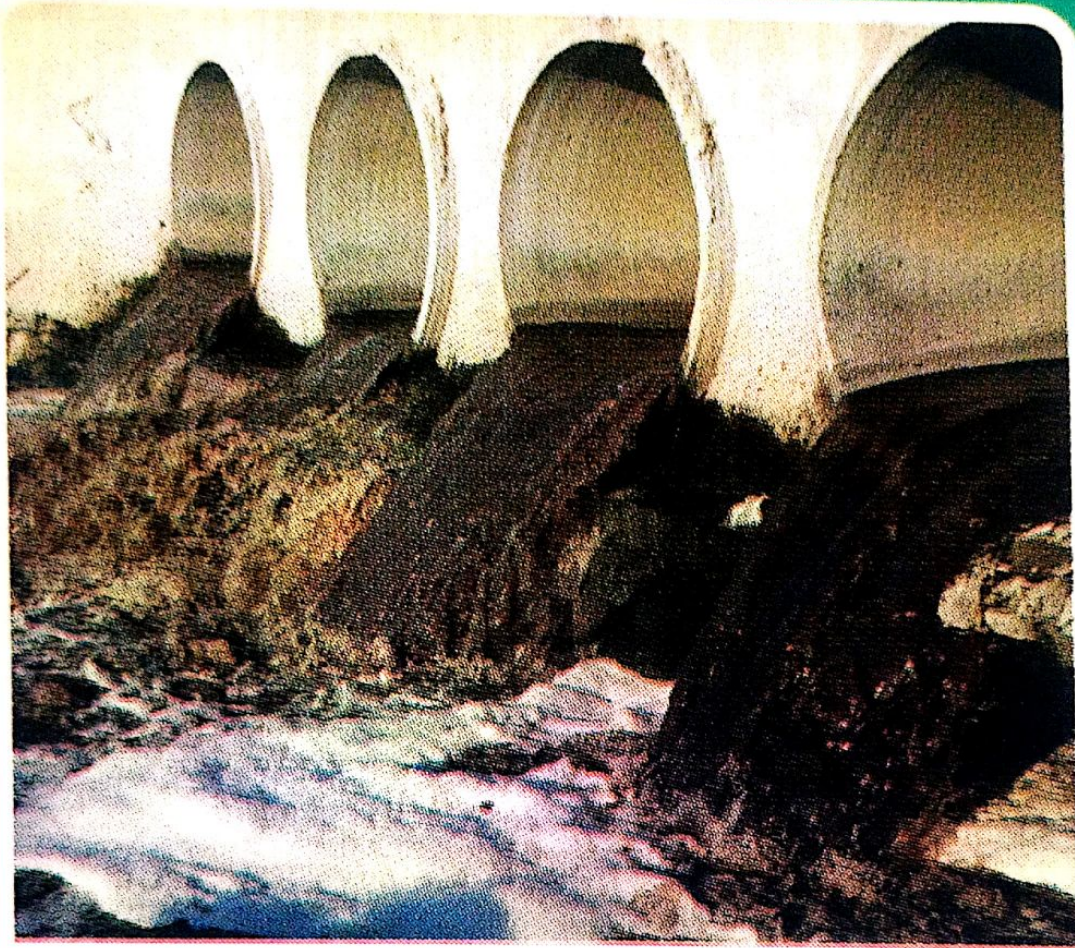
WATER POLLUTION - IMPROPER ORAINAGE
